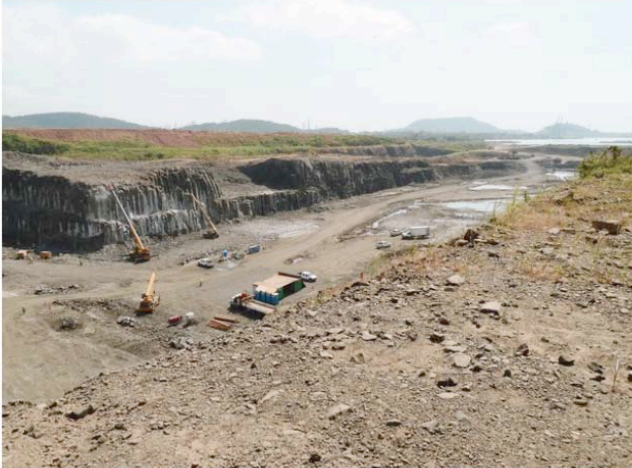
New locks were under construction at the Panama Canal in February. The twin ports of Los Angeles and Long Beach could lose as much as a quarter of their cargo business by some estimates after the Panama Canal expansion is completed in 2014. (AFP/Getty Images / February 9, 2011)
