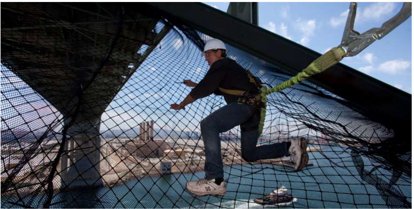
Protective netting (known as a “diaper”) under the bridge catches falling pieces of concrete and requires regular maintenance.
